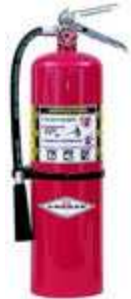
4A rated extinguisher. Sufficient fire protection.
